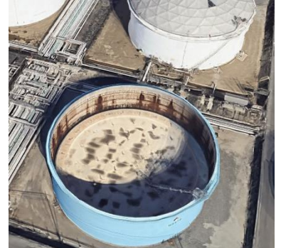
EXTERNAL FLOATING ROOF
